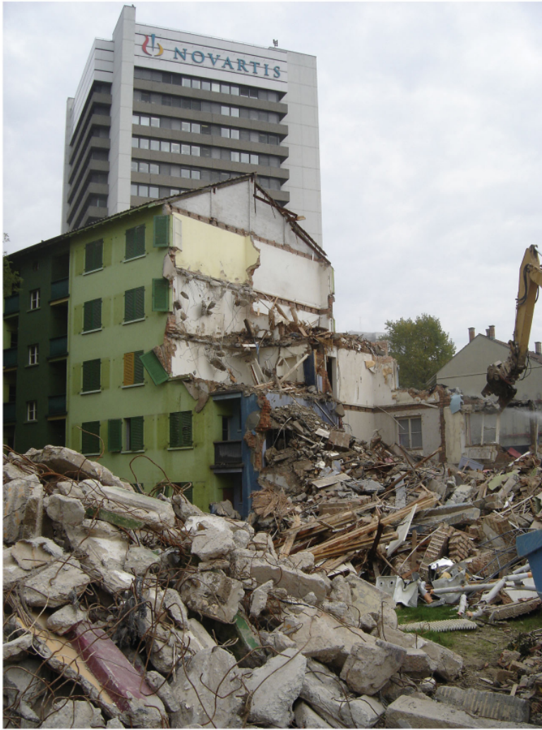
Figure 3 Demolition of apartment blocks known as the “Papageienhäuser,” in Bruchstücke Basel Nord, 2009, 1. (Photo Ali Meraihia)
